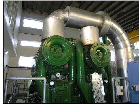
Original diesel engine driving the pumps
