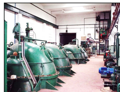
Original pumps installed by W H Allen
