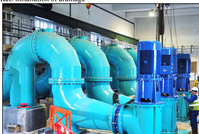
Bedford Pumps' installation at Welches Dam P.S.
