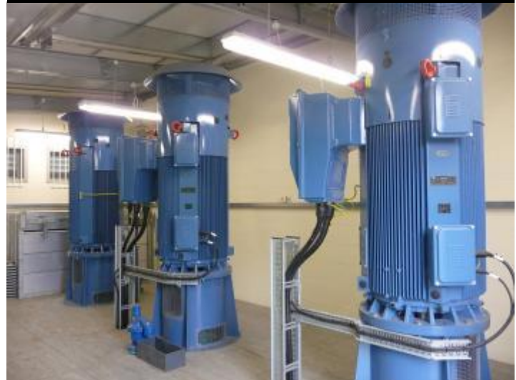
Bedford Pumps' suspended Bowl Pumps
