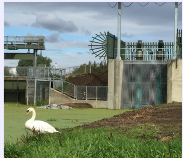
Webb's Hole pumping station
