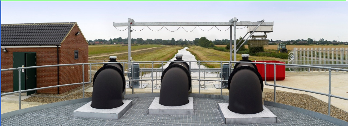
Puny Drain Pumping Station
