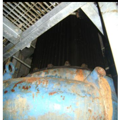
Rotating element with existing pump casing installed at Black Rock P.S.
