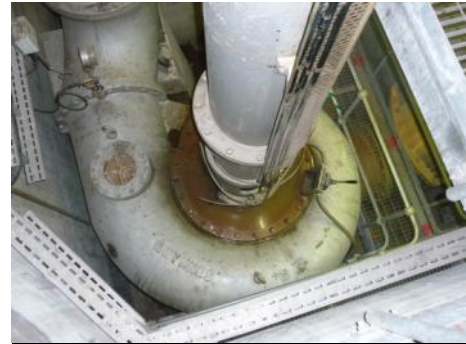
Existing Allen Gwynne pump installed at Netheridge
