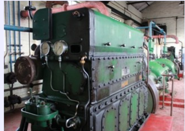
Diesel engine driving the old pumps at Cam Pumping Station
