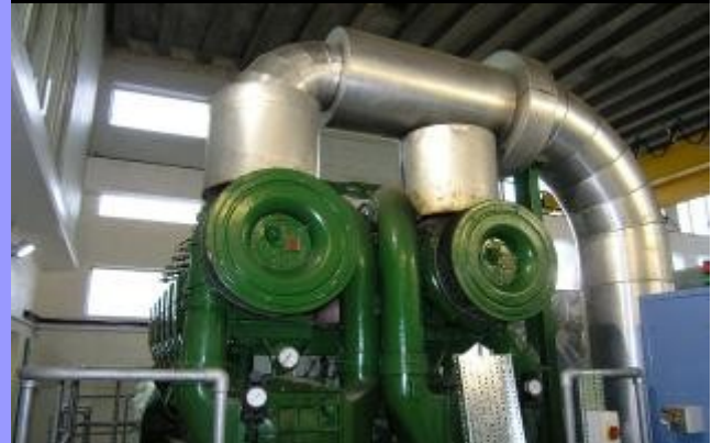
Original diesel engines driving the pumps
